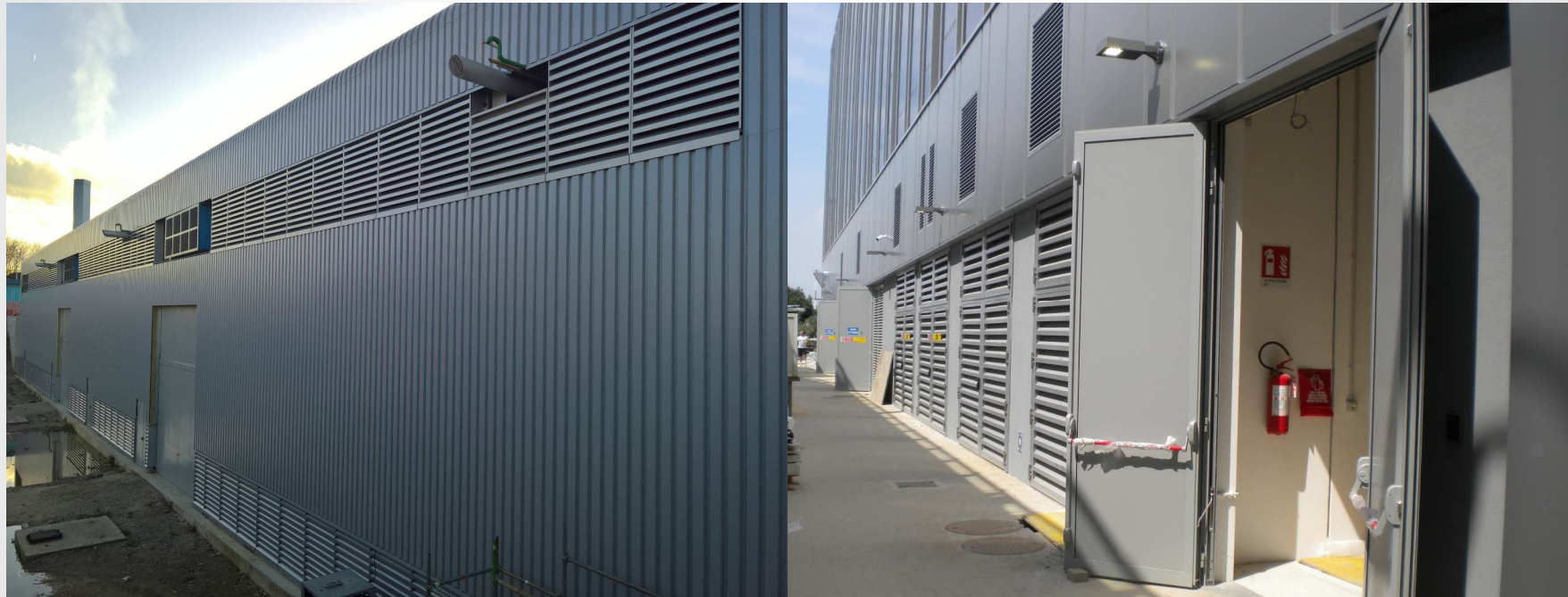
Thermal power station A2A – Brescia Acoustic grilles
